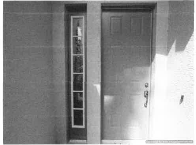
Front unprotected door
