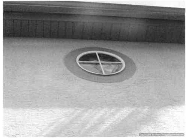
Left unprotected window
